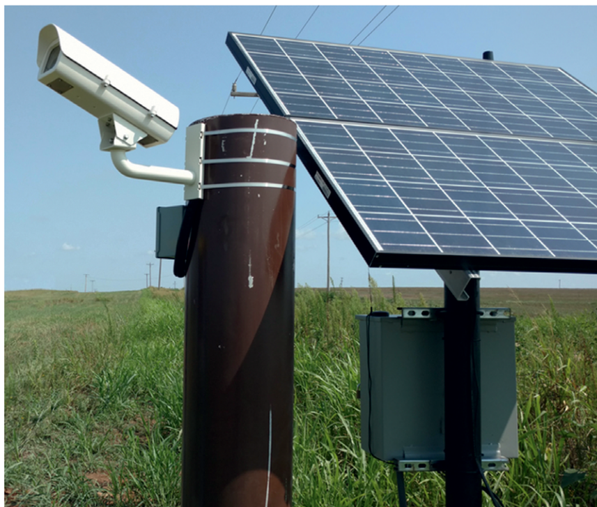
FIG. 4. One of the six cameras that compose the stereo ring. The pole-mounted camera, tilted approximately 18° from the ground, is powered by two solar photovoltaic panels connected to a lead-acid battery and communicates with the ARM servers using a cellular network.
